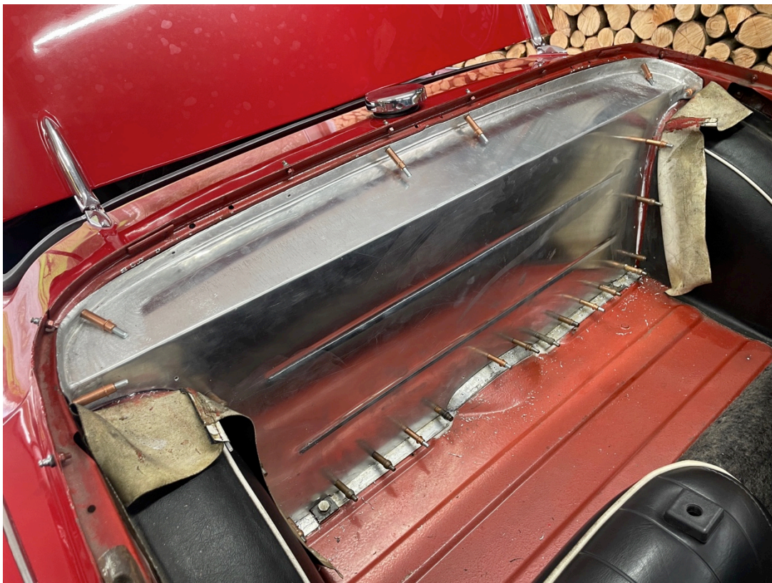
Firewall held in place with Cleco pins while being drilled for final riveting
