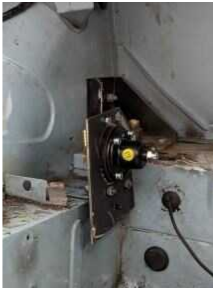
New PRV in the boot beneath the tank (not yet installed here)
